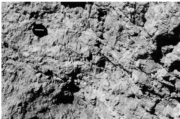
Fig. 4 Strongly altered Silurian limestone that shows evidence of both transitional and chalky zone alterations. Note that the chalky development first appears along the bedding planes (light inclined stripes) whereas rusty yellow rock in between still exhibits somewhat lower degree of decay. Plant roots penetrate the rock along the system of sub-vertical fractures. Lobolitová stráň Hill near Řeporyje.
